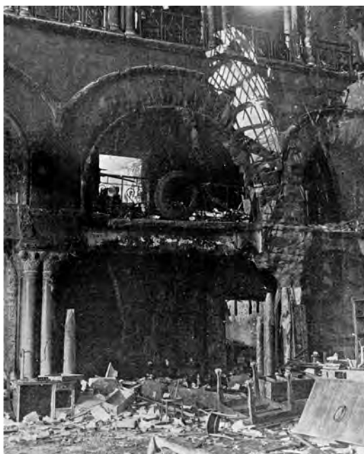
Central Reading Room after the fire
