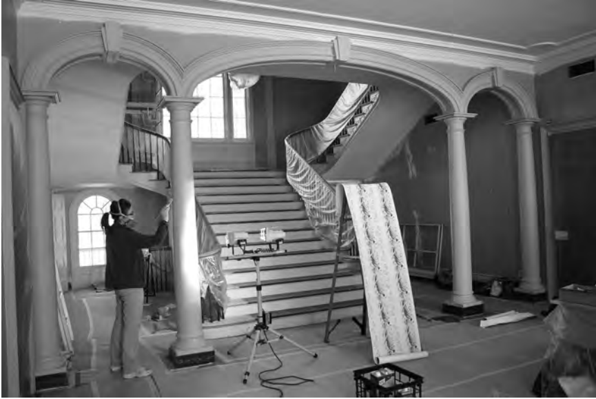
Painting trim elements with handmade pigmented linseed oil paint is conservation technician, Nicole Sequin during 2014 historical upgrade of the entrance hall
